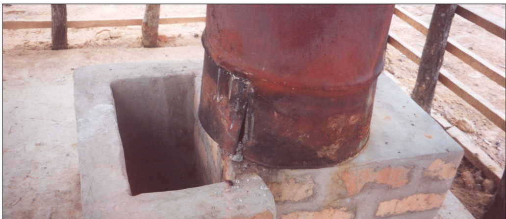
Oil drum burner, Zambia
