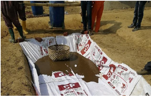
Infiltration bed (with basket to filter out plastic waste) rain)
