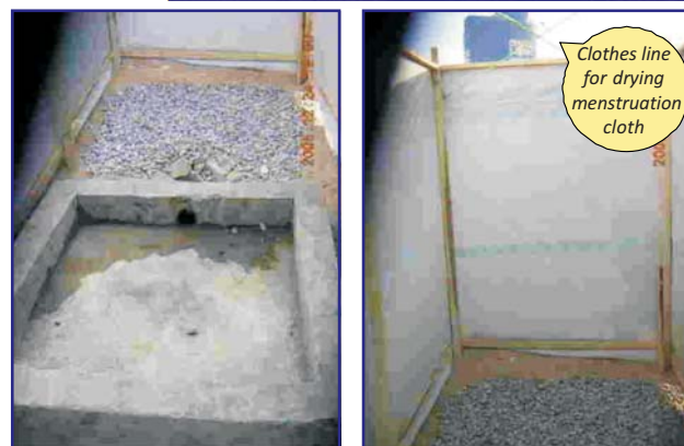
Washing slab for menstrual cloths inside a screened block and washing lines for drying the cloths
