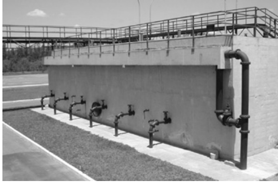
Figure 27.10. View of a full-scale UASB reactor Source: Ipatinga WWTP, COPASA, Brazil
