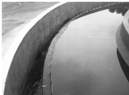
Figure 27.19. Effluent collection device (plate with V-notch weirs) Source: Nova Vista WWTP, Itabira, Minas Gerais, Brazil
