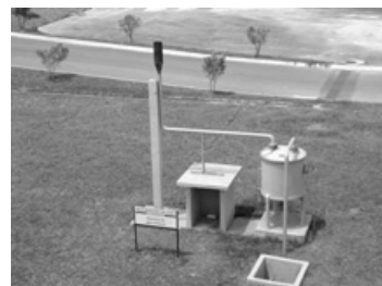
Figure 27.21. View of a hydric seal and gas burner (source: Ipatinga WWTP, Minas Gerais, Brazil)
