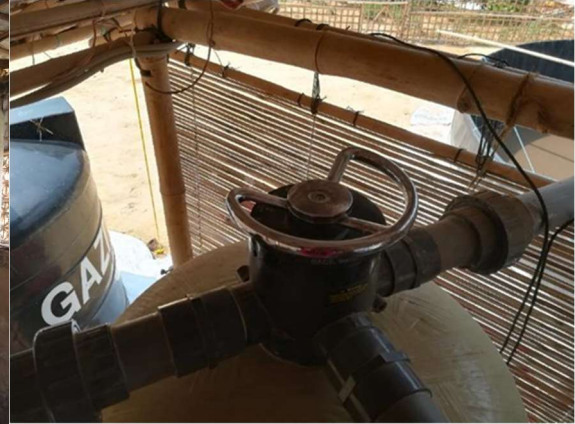
Picture 12: Filter operation valve
