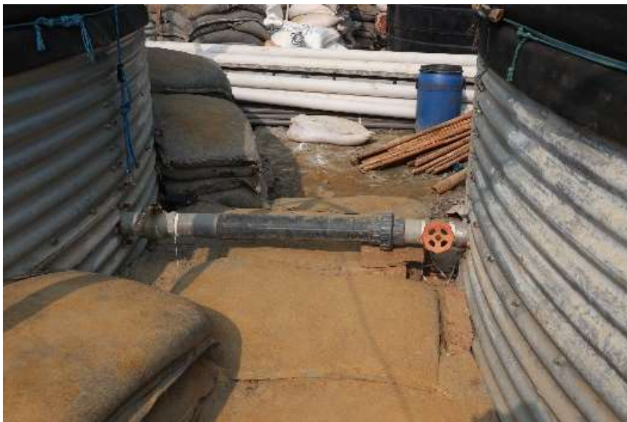
Picture 9: Gravity valves
