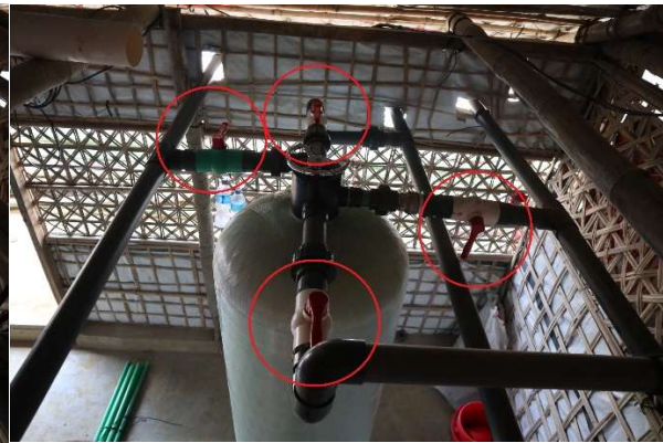
Picture 16: Valves set on “Filtration”
