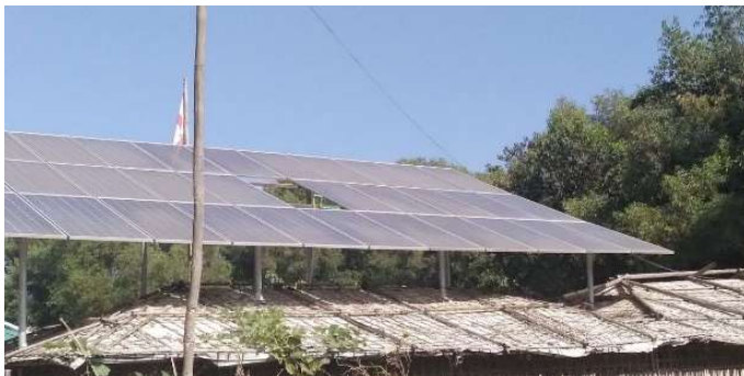
Picture 2: Dust on the solar panels
