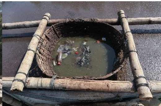
Picture 3: Dirty inlet screen
