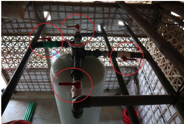
Picture 15: Valves set on “Backwashing”
