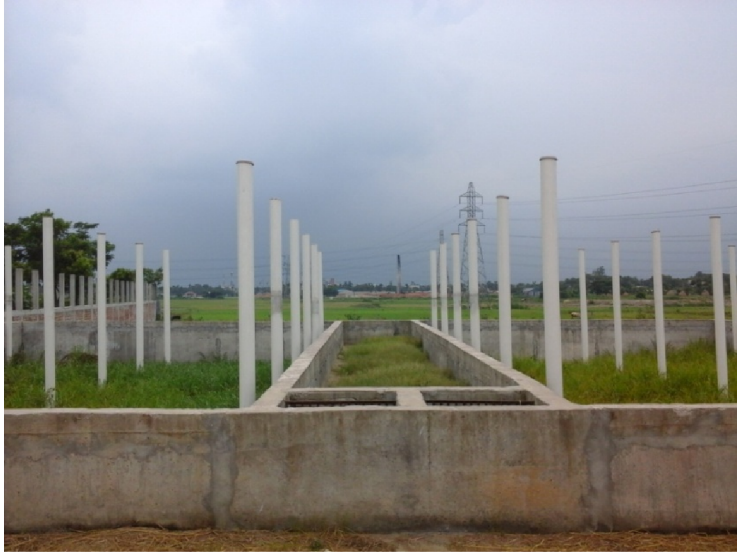
Figure-2a: Planted sludge drying bed of FSTP at Narsingdi Pourashava, Bangladesh
