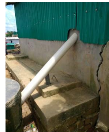
Example of latrine equipped with chute for discrete disposal of MHM material (PVC pipe connected to a sealed pit) (Source: IFRC/Swedish Red Cross)
