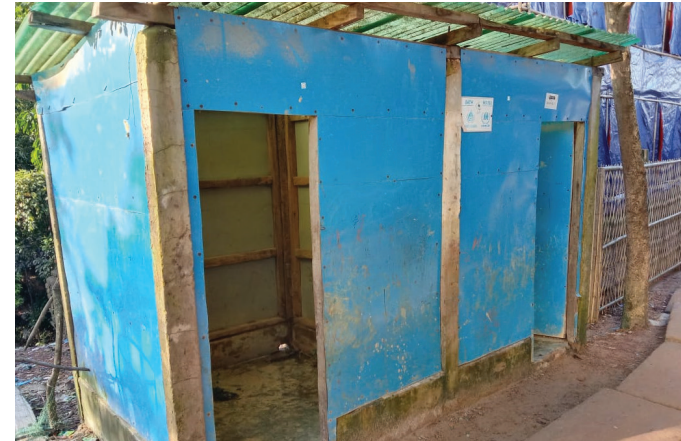
Figure 33: Multiple cubicles bath house (Courtesy: UNHCR)
