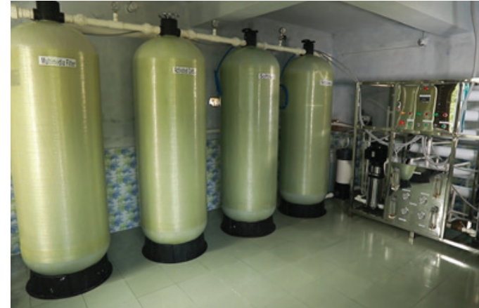
Figure 20: Reverse Osmosis (RO) plant (Courtesy: DPHE)
