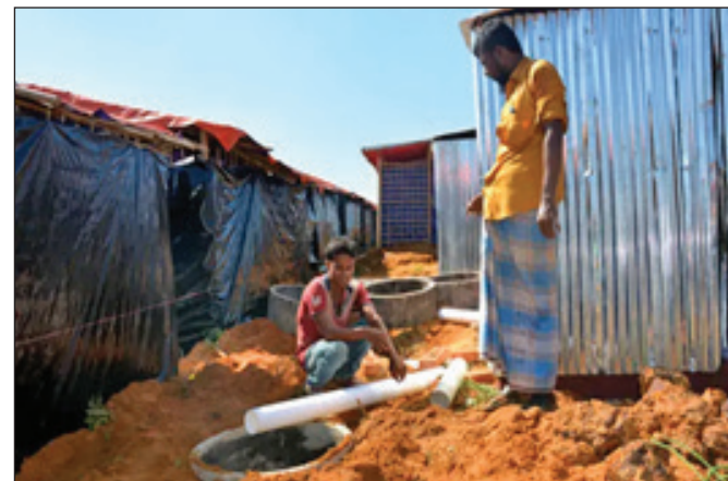
Figure 26: A multiple cubicle twin pit latrine in construction in Cox's Bazar (Courtesy: Devex)
