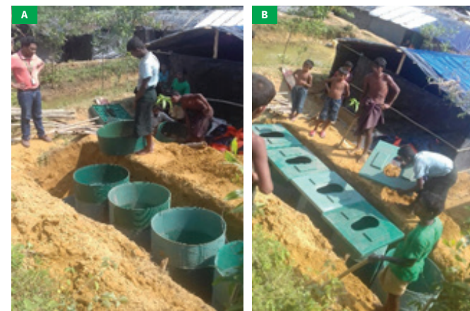
Figure 11: A. Positioning of plastic rings; B. Placing of Plastic slabs of a plastic communal latrine (Courtesy: Oxfam)
