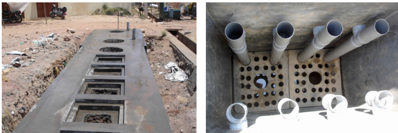
FIGURE 7: AF baffles with inlet and outlet pipes (left); up- and down-flow pipes. [8]
