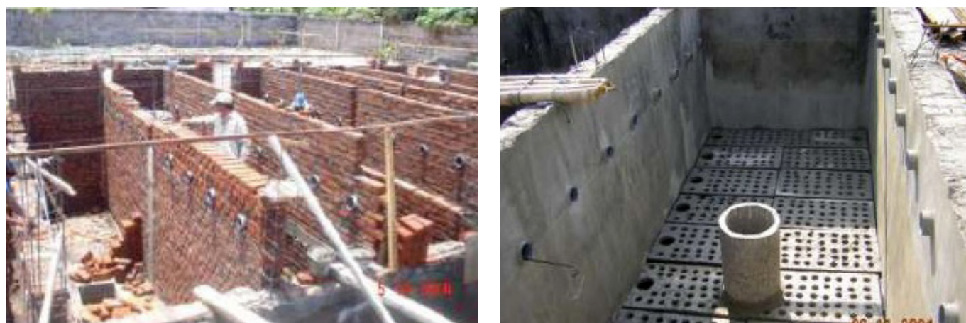
FIGURE 6: During construction: view of an AF (left) and slabs to support the filling media with a central concrete nozzle for desludging (right). [7]
