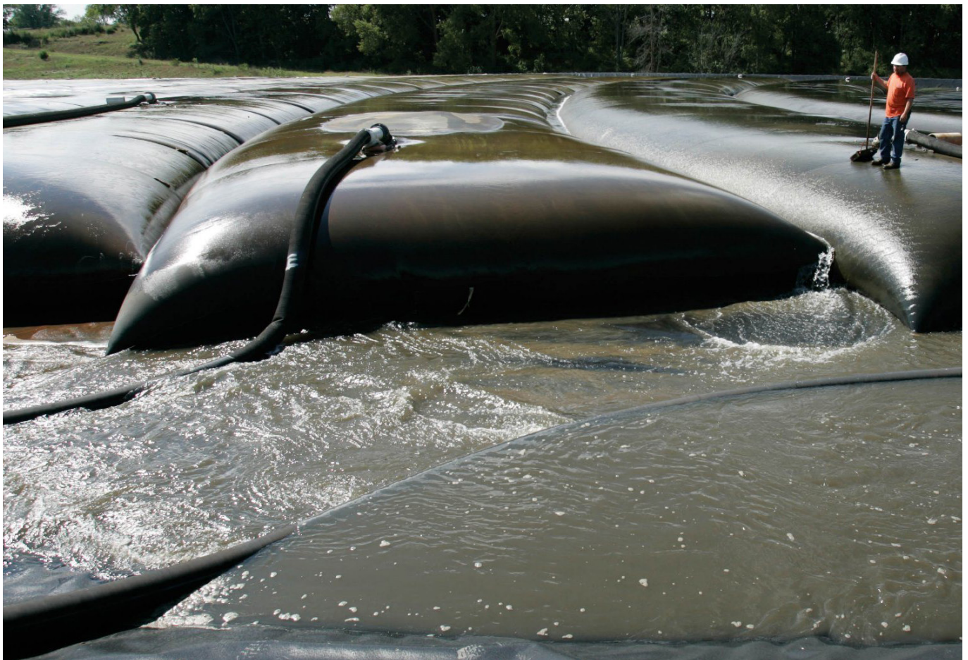
FIGURE 11: Geotubes for sludge thickening.
