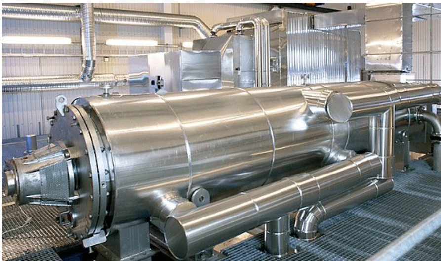
FIGURE 35: Technical installation for thermal drying of sludge.
