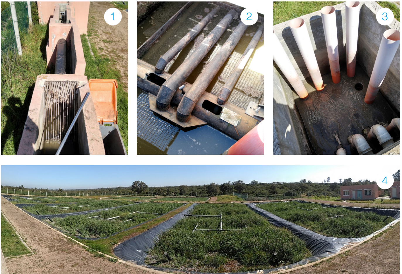
FIGURE 67: Tidili, Morocco: Wastewater treatment chain including vertical filter cells: (1) Screening, (2) “Siphon”, (3) Distribution system / “Valves”, (4) Vertical filter cells. [60]
