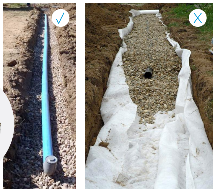
FIGURE 80: Illustration of French drain slope; geotextile is not recommended for wastewater (risks of cloggings). [73]
