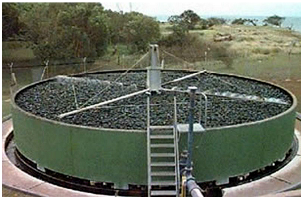
FIGURE 27: Example of a cylindrical trickling filter (left). [28]
