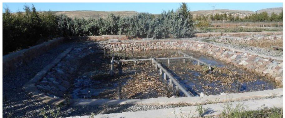
FIGURE 68: Tidili, Morocco: Horizontal filter cells as integrated part of the wastewater treatment chain. [61]
