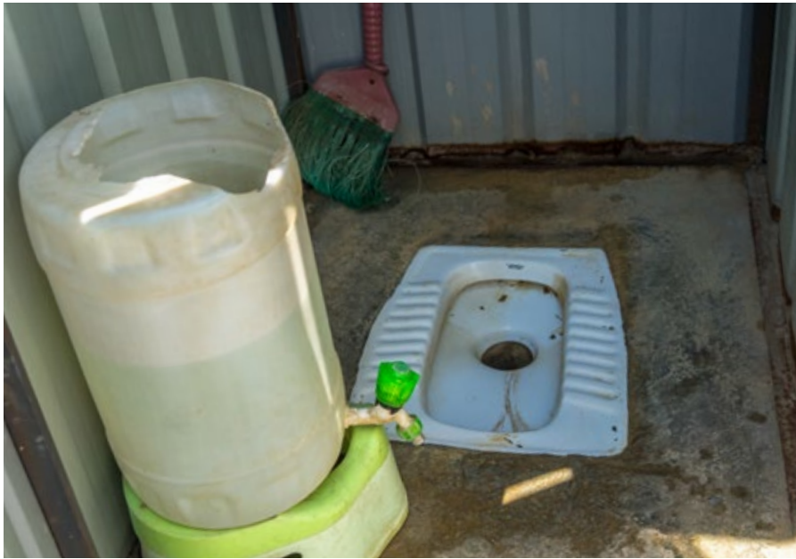
FIGURE 4: Typical pour flush toilet installed in the shelter. Water container for anal cleaning and hand washing. Broom in the back for cleaning.
