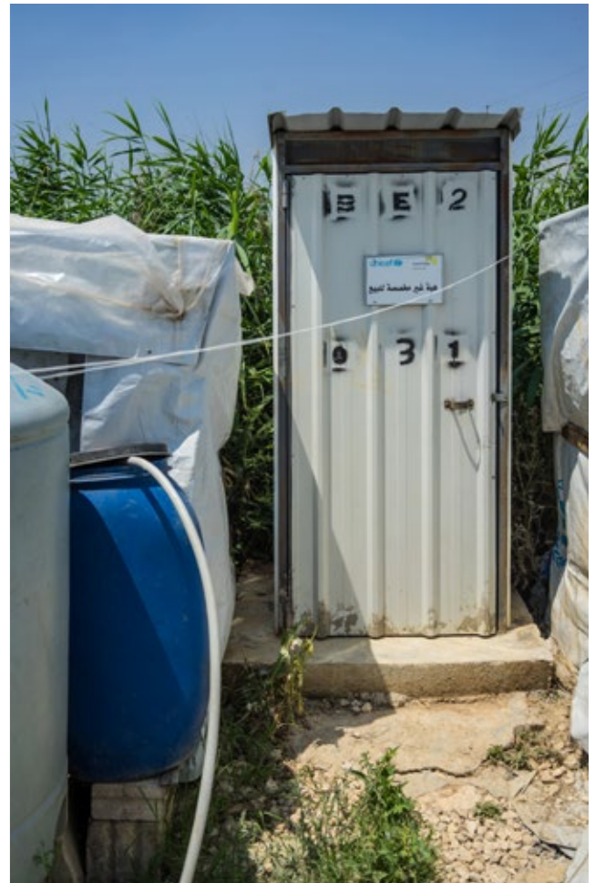
FIGURE 3: The toilet is installed in a corrugated tin roof shelter. The holding tank is located under the concrete platform.
