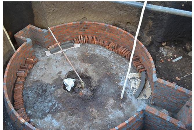
FIGURE 23: Bottom of biogas plant with in- and outlet shafts.
