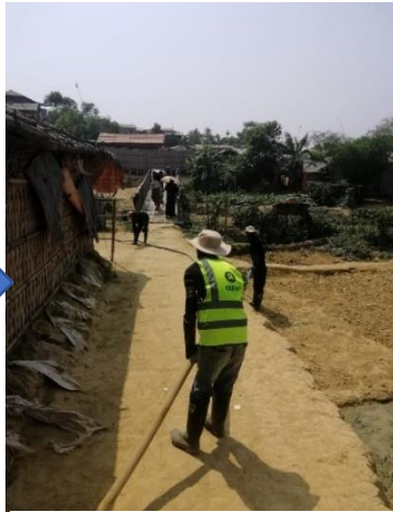
Figure 1: Pumping to nearest transfer station or Transfer Pit.
