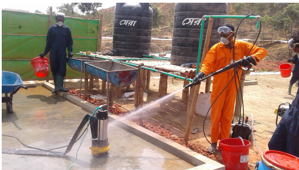
Figure 16: A staff member is cleaning a submersible pump with a high-pressure device at the faecal sludge treatment plant in Cox's Bazar, Bangladesh (source: Marij Zwart)
