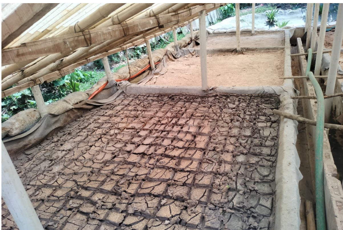
Figure 15: An unplanted drying bed loaded with faecal sludge in Cox's Bazar, Bangladesh (source: UNHCR).
