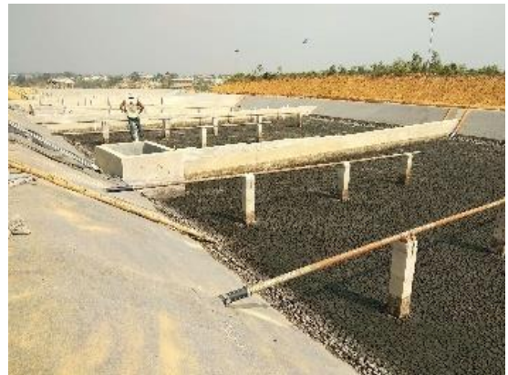
Figure 3 : Planted Drying Bed ,Year 2020
