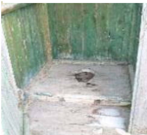
Photo 3.7 Pit Latrine with Improved Slab
