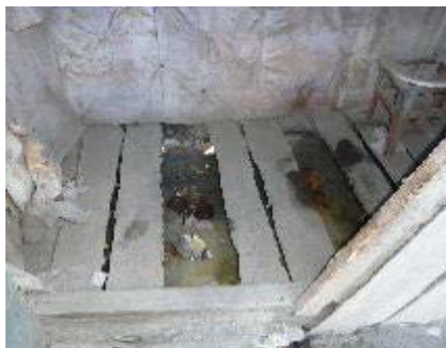
Photo 3.6 Unimproved Basic Pit Latrine
